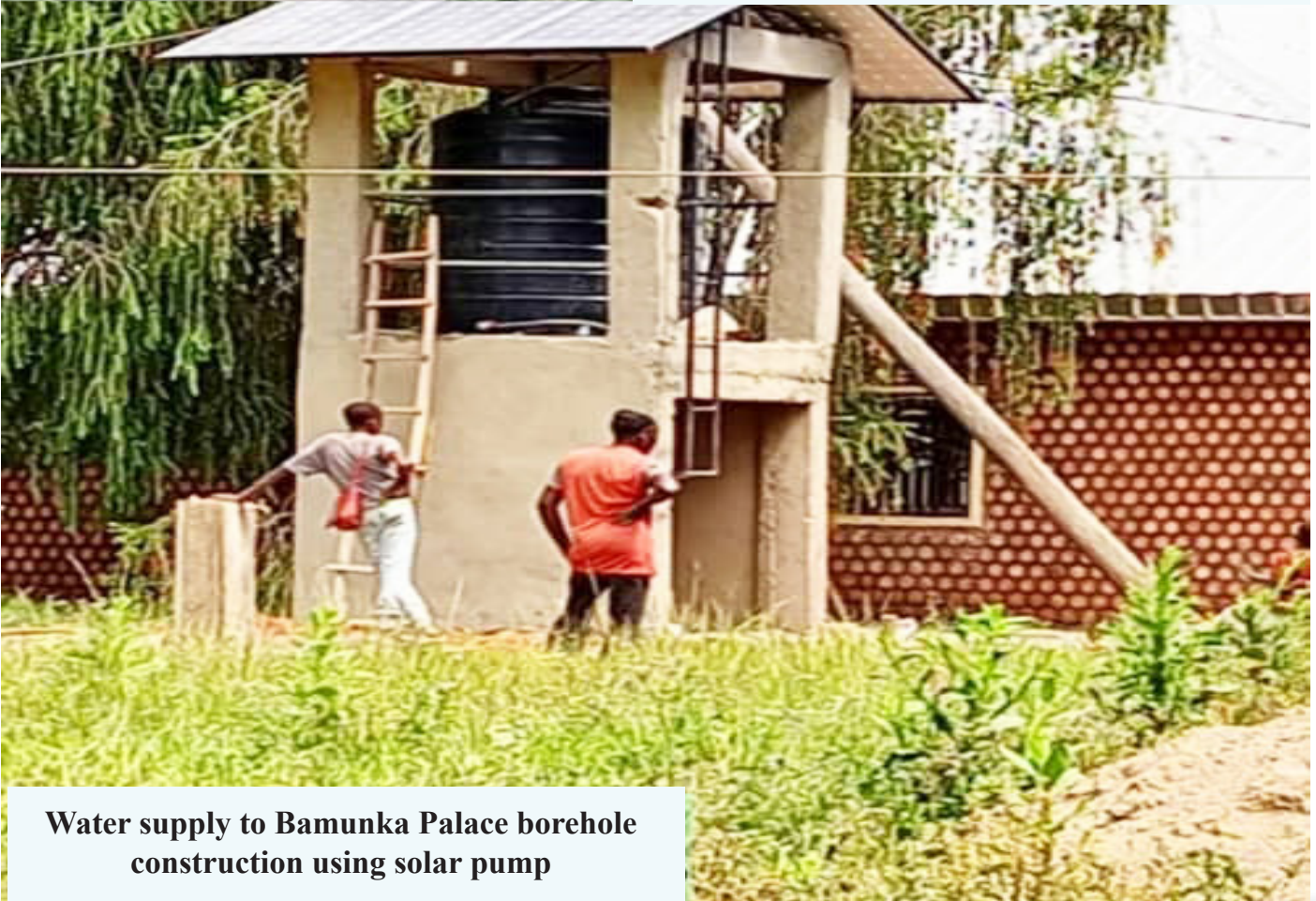
Work progress during the construction of the borehole at Bamunka Palace in Ngoketunja Division
