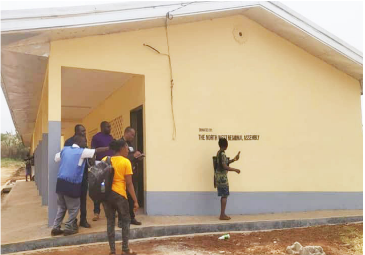
Construction of a block of 2 classrooms and 4 compartment squatting toilet at CCAST Bambili
