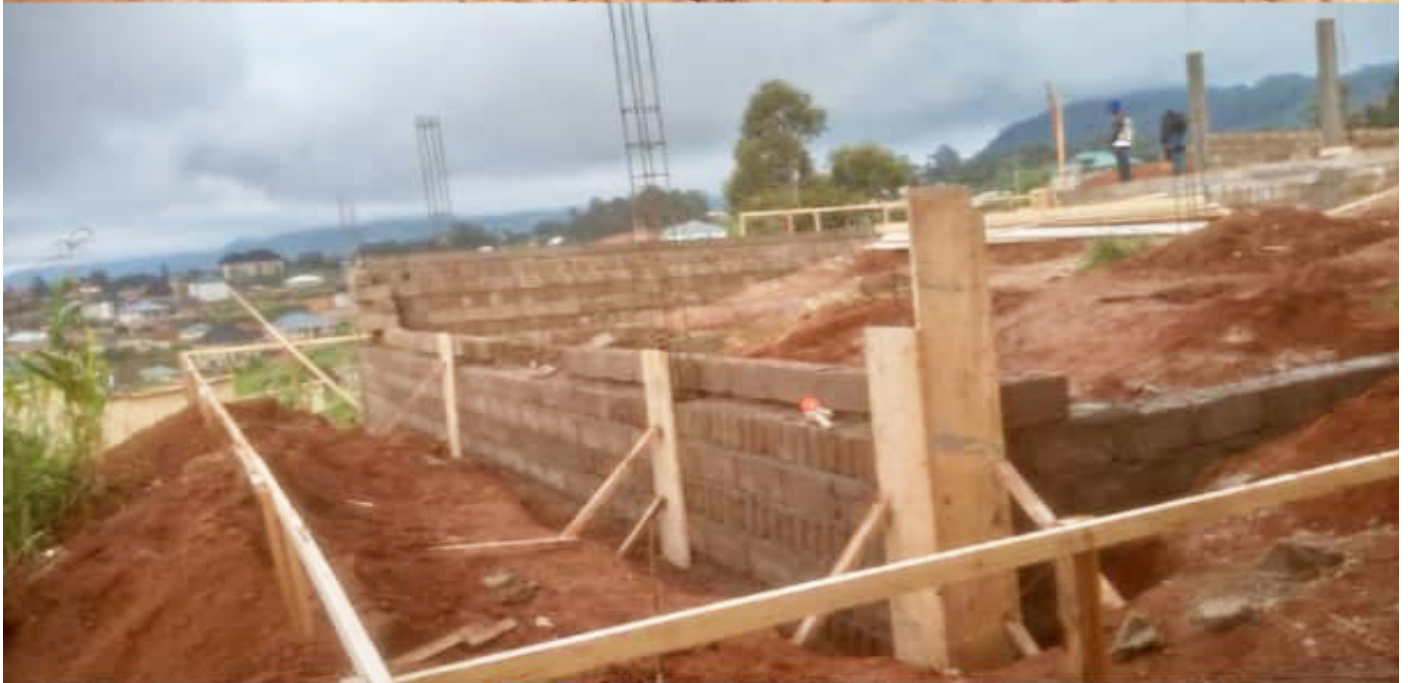
Construction of a multipurpose laboratory at GBHS Bamendankwe – Excavation before work commencement
